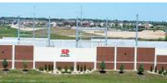
Utilities (SPU Substation)
