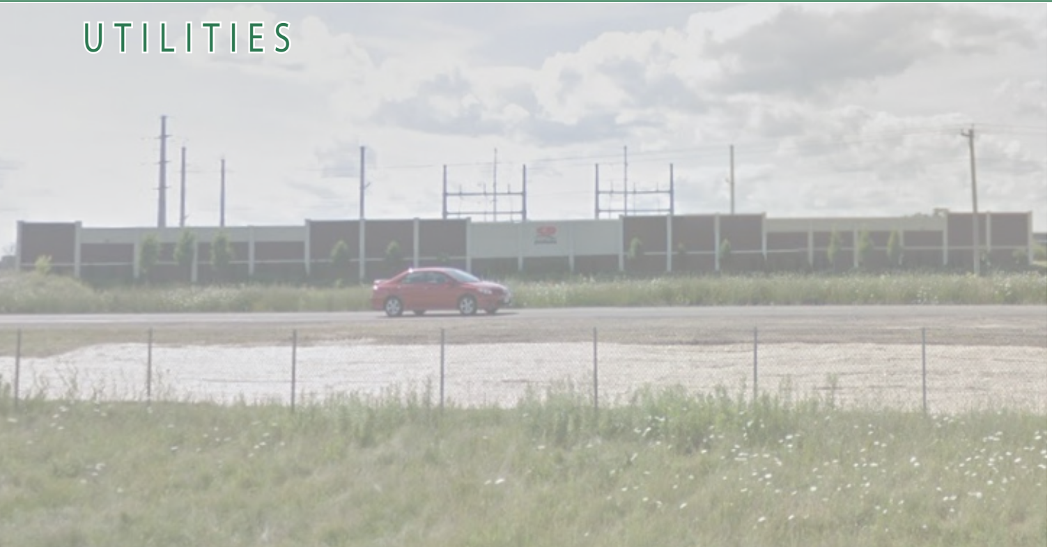
Sun Prairie HWY 151 Substation
