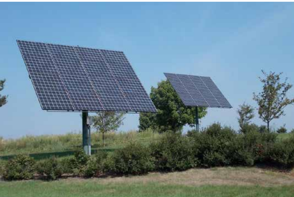
WPPI Solar Panels in Sun Prairie Business Park
