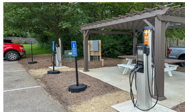
EV Charging Stations, City Hall
